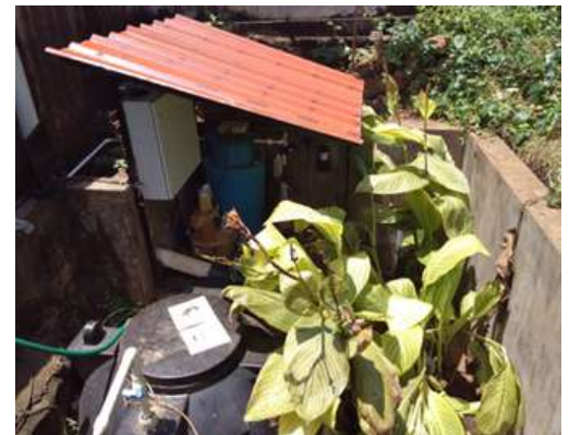
Wastewater Treatment Plant
